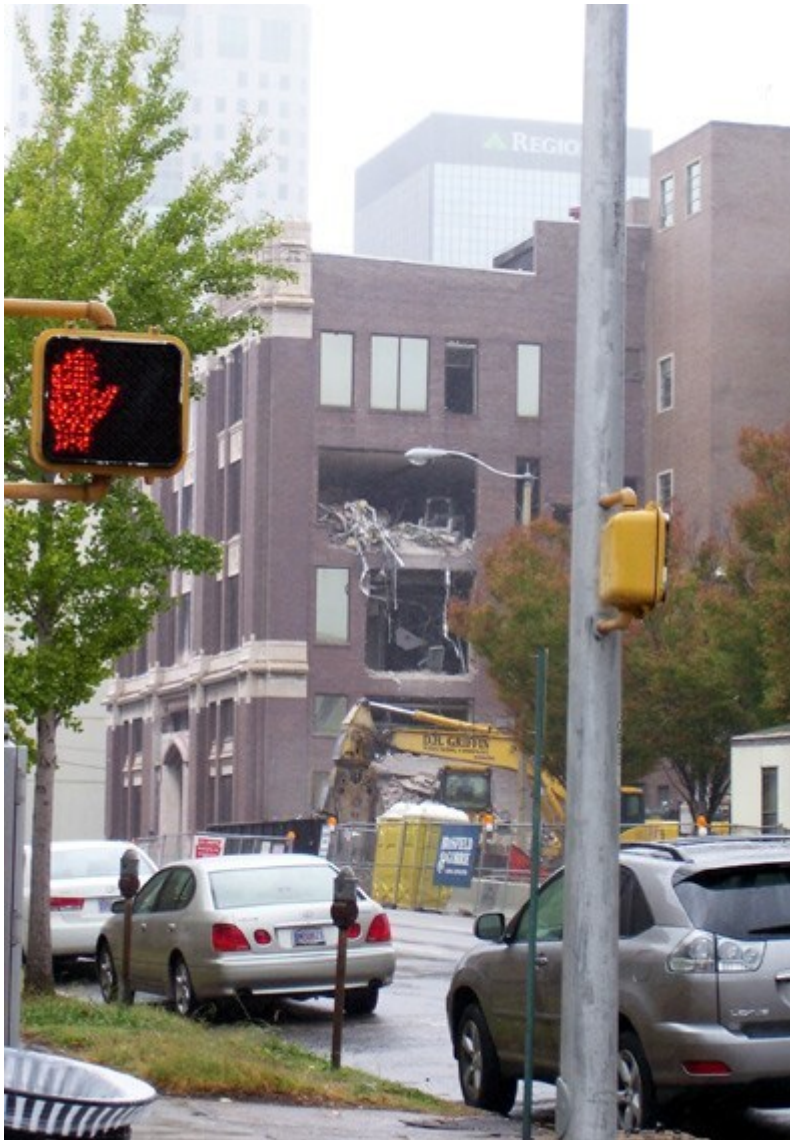
Holes have been punched high on the eastern wall of the Birmingham News' original 1917 structure as its demolition continues. Photo credit: André Natta
